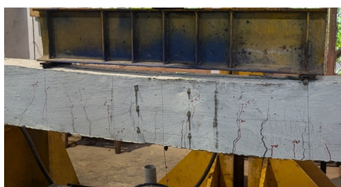
Fig 6. Failure Pattern of ECFS Beam
