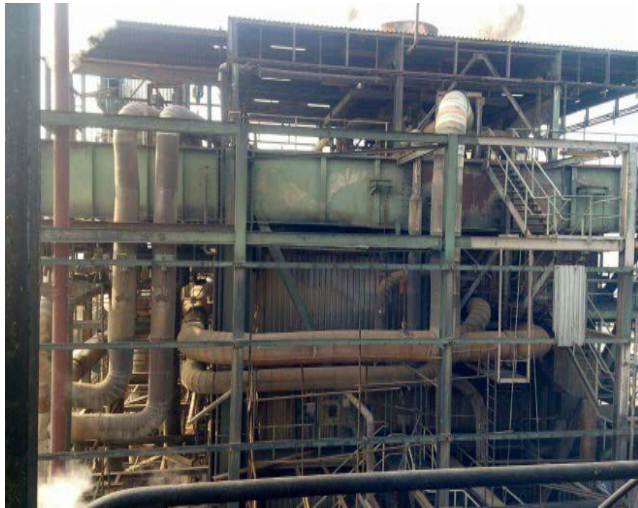
Figure 1. Steam boiler in power plant AL – Dura.
