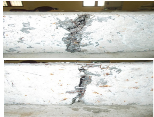
Figure 5. Crack patterns of specimens after failure.
