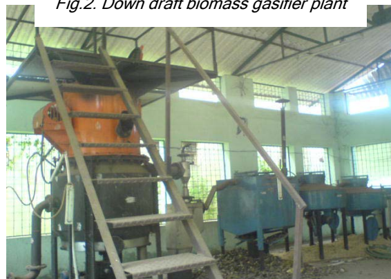
Fig.2. Down draft biomass gasifier plant
